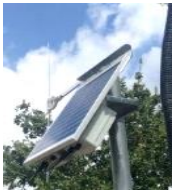
PR-00006. DrainVision Base station solar powered.
