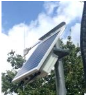
PR-00006. DrainVision Base station solar powered.
